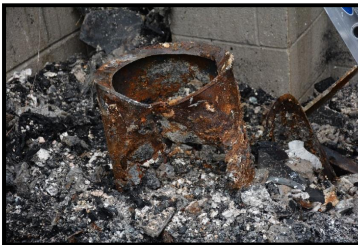
Figure 10 – Damaged ceiling light can
